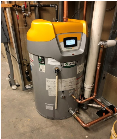
Figure 2.1 High Efficiency Hot Water Tank at Health Services Building
