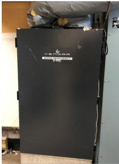
Figure 2.3 Heat Recovery Ventilator (HRV) at the Municipal Offices
