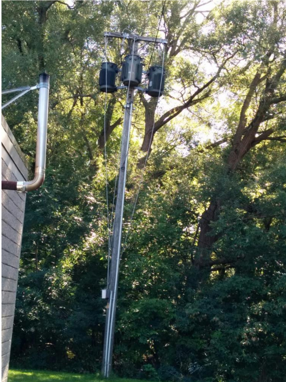
ID01_E04: Old Service Transformers
