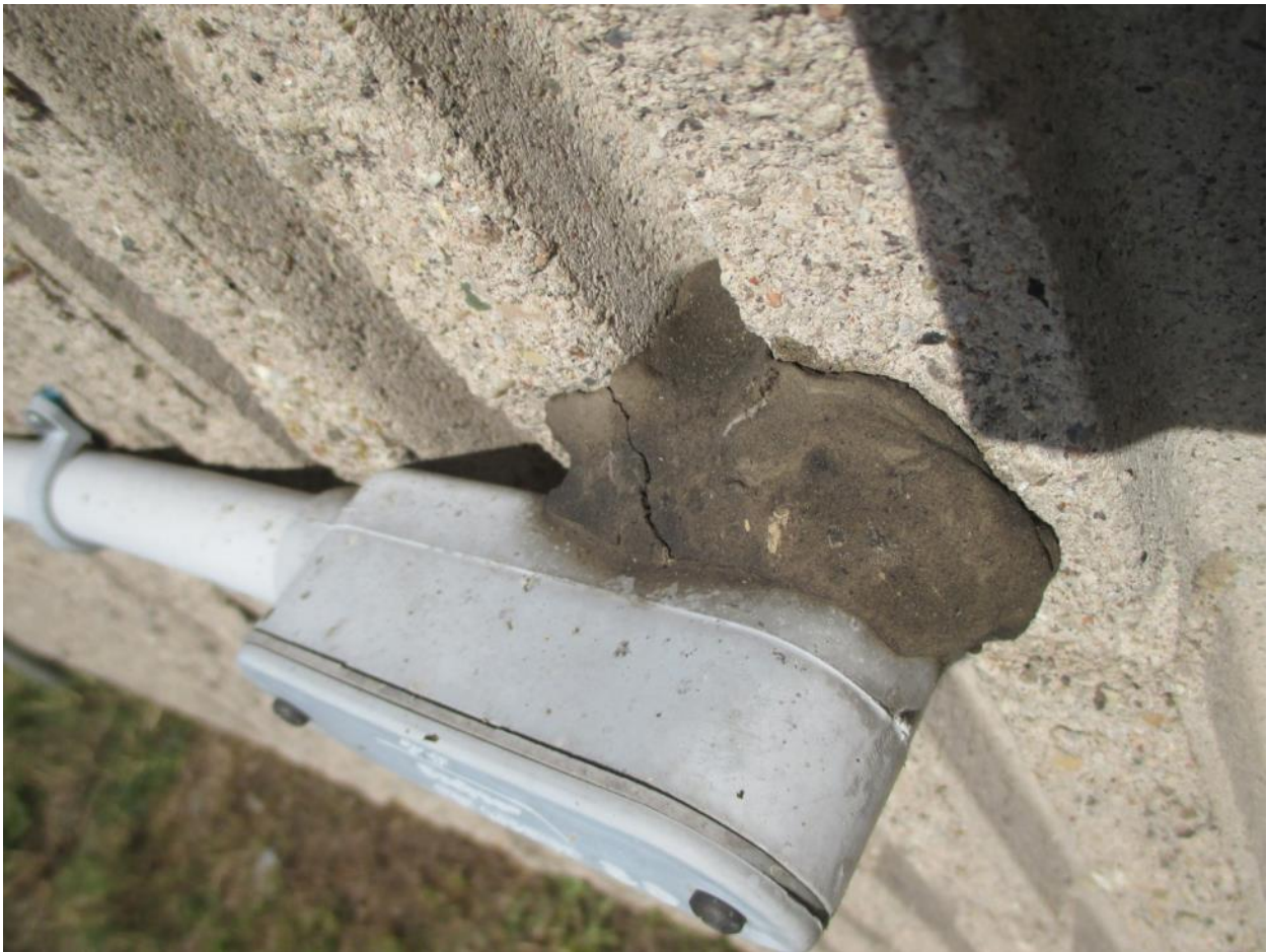
ID02_AS06: Brittle and Cracking Seal
