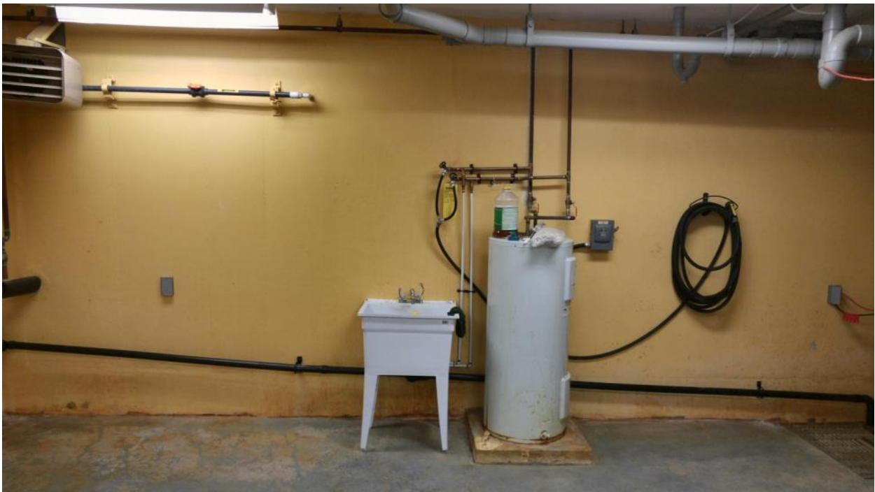
ID02_M02: Corrosion at the Base of the Hot Water Heater
