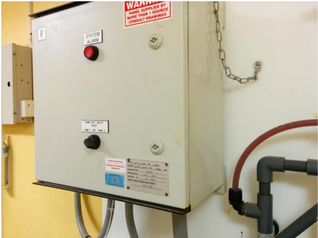
ID02_E04: Ferric Chloride Control Panel
