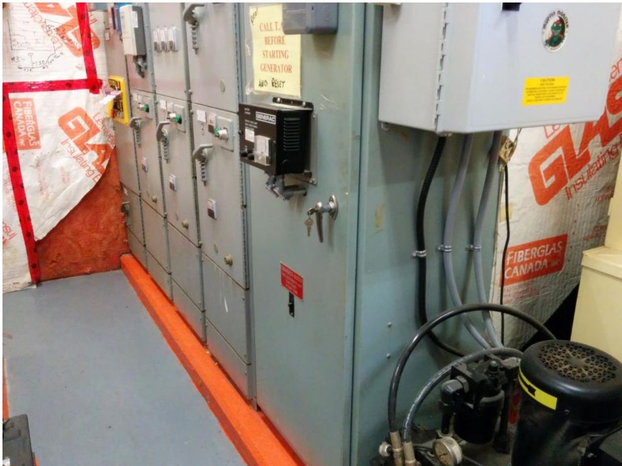
ID01_E03: Clearance between MCC and Generator Battery
