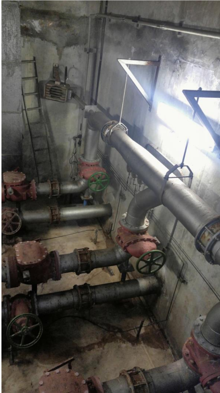
ID01_M04: Rusted Piping in the Dry Pit
