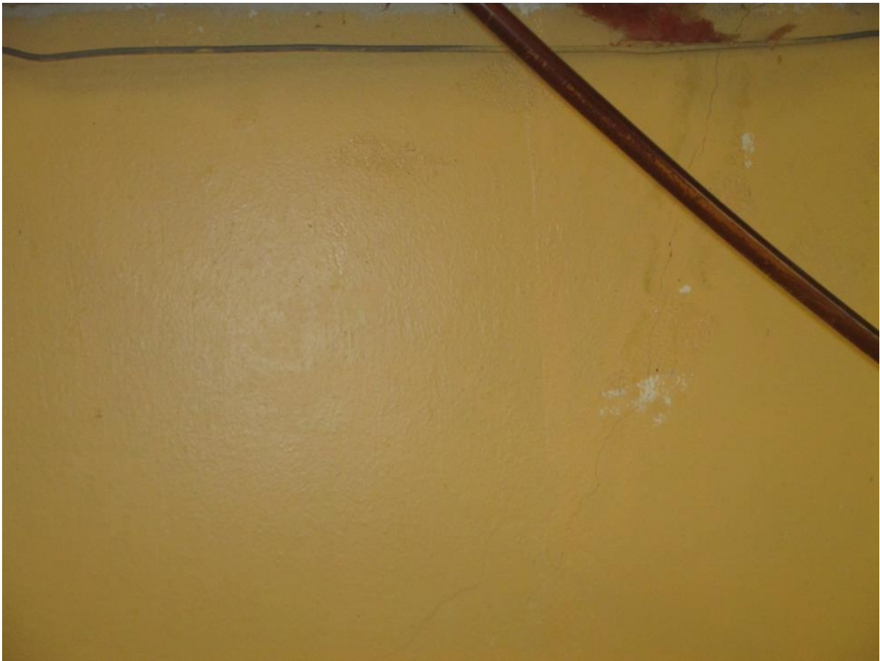
ID02_AS03: Crack in Basement Wall
