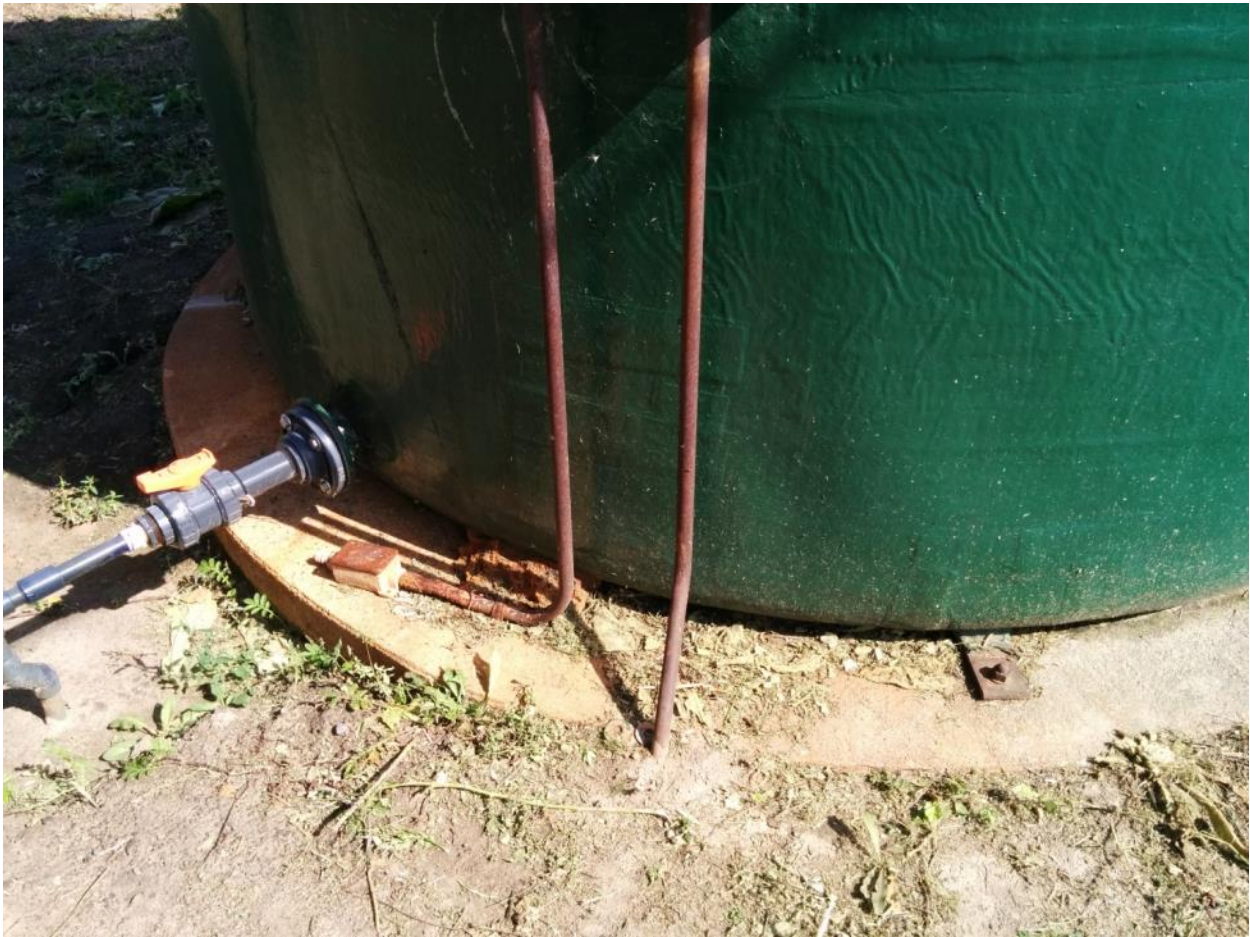
ID02_E01: Corroded Conduits to Ferric Chloride Tank
