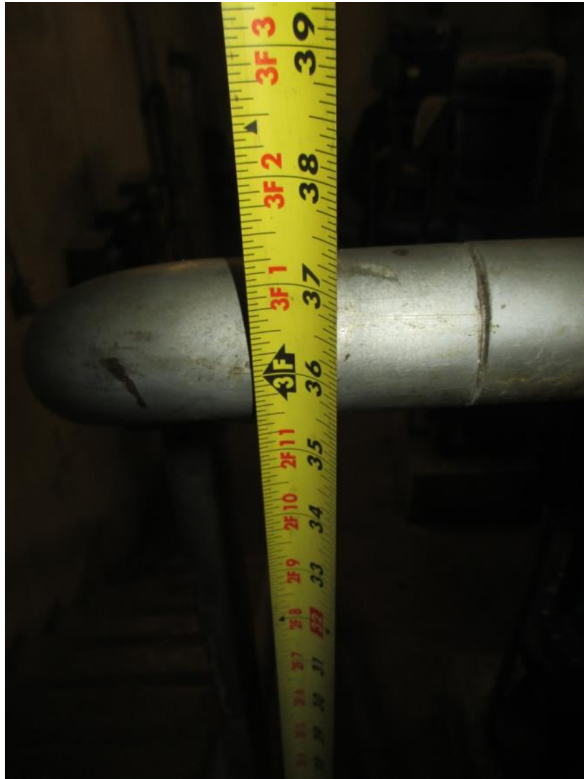
ID01_AS12: Insufficient Guardrail Height
