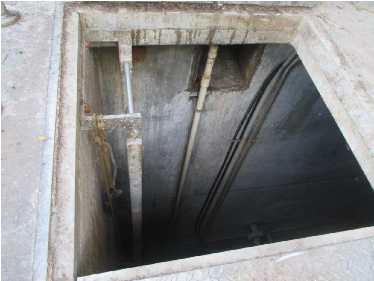
ID01_AS06: Ferrous Fasteners on Aluminum Access Ladder
