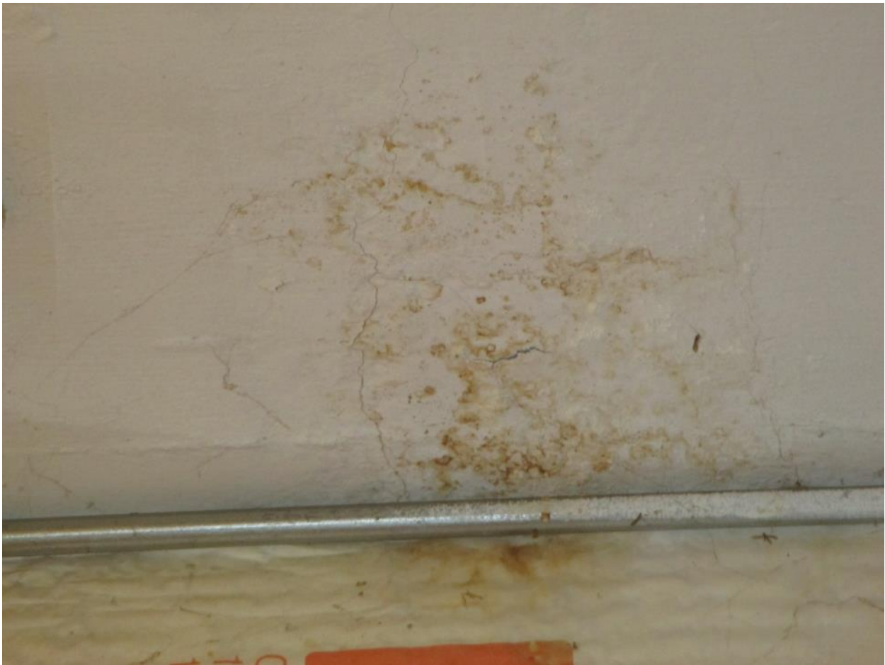
ID01_AS07: Paint Coating Damaged by Water
