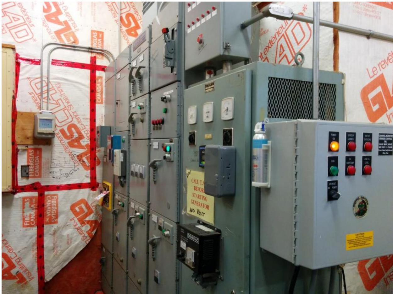
ID01_E06: MCC and ATS
