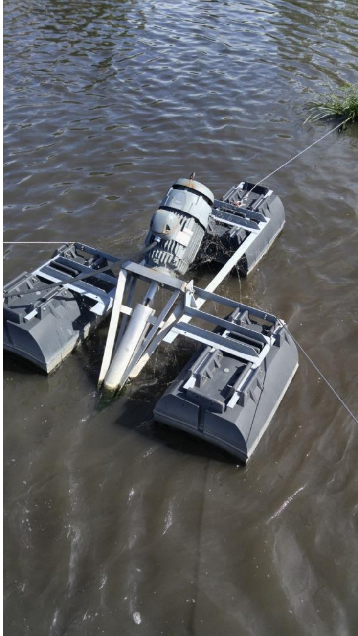
ID02_M04: New Mechanical Aerators
