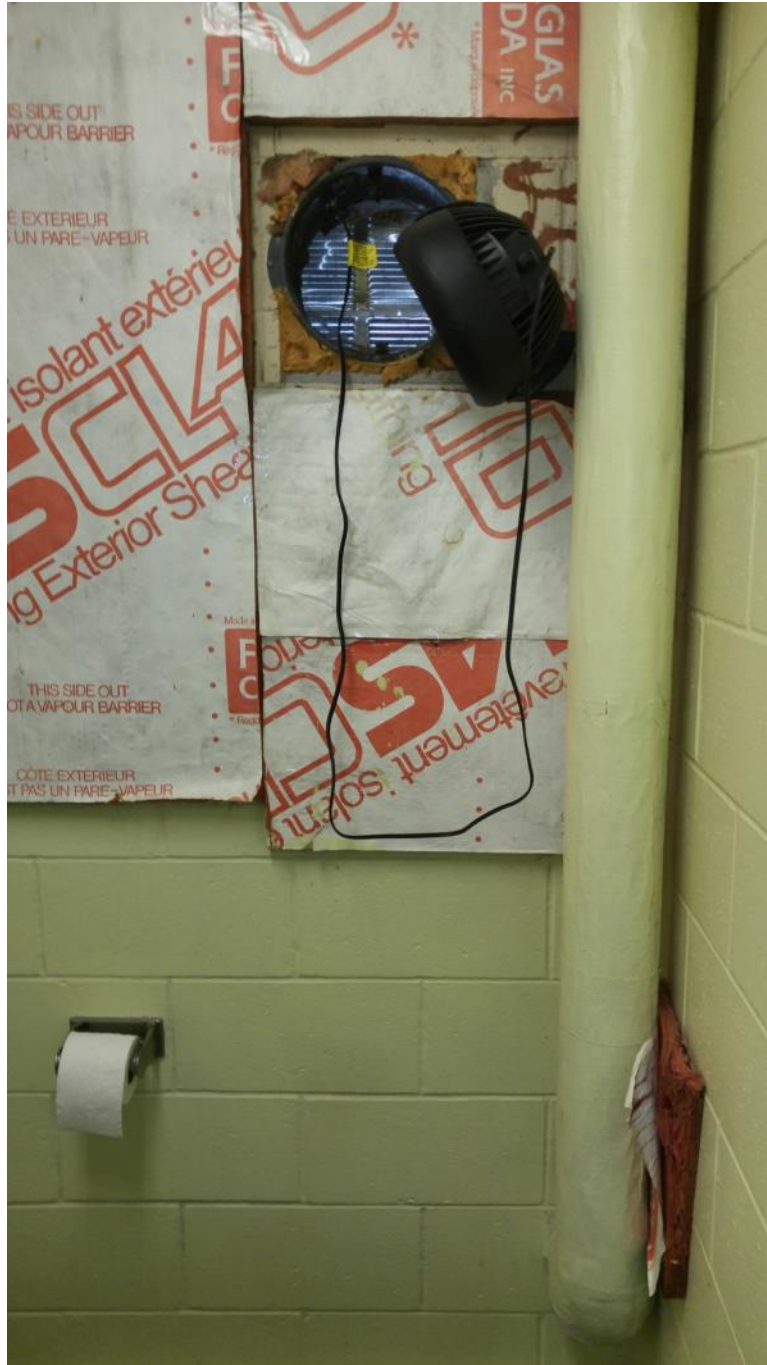
ID02_M01: Washroom Exhaust Fan
