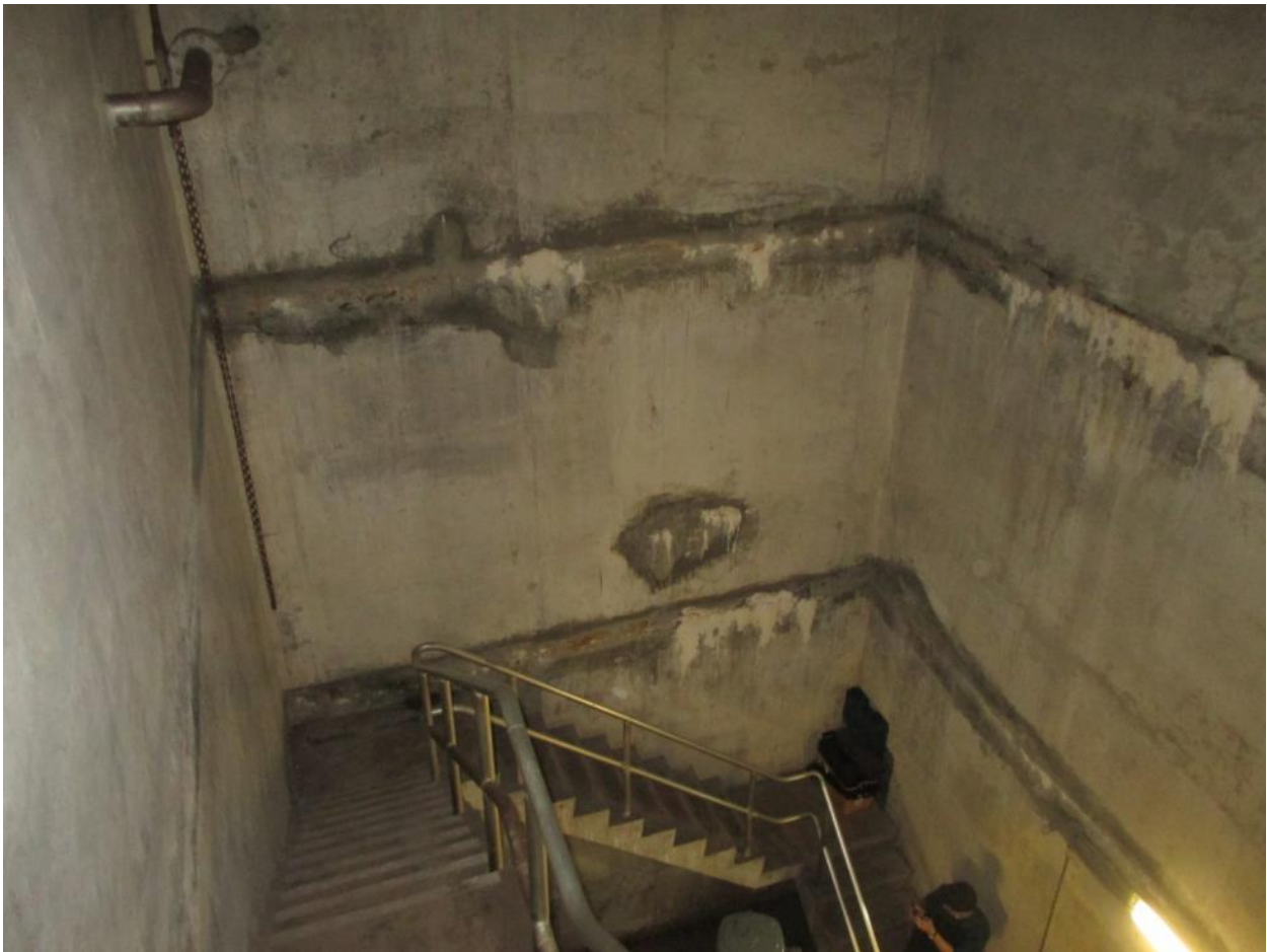
ID01_AS02: Water Damage and Concrete Repairs
