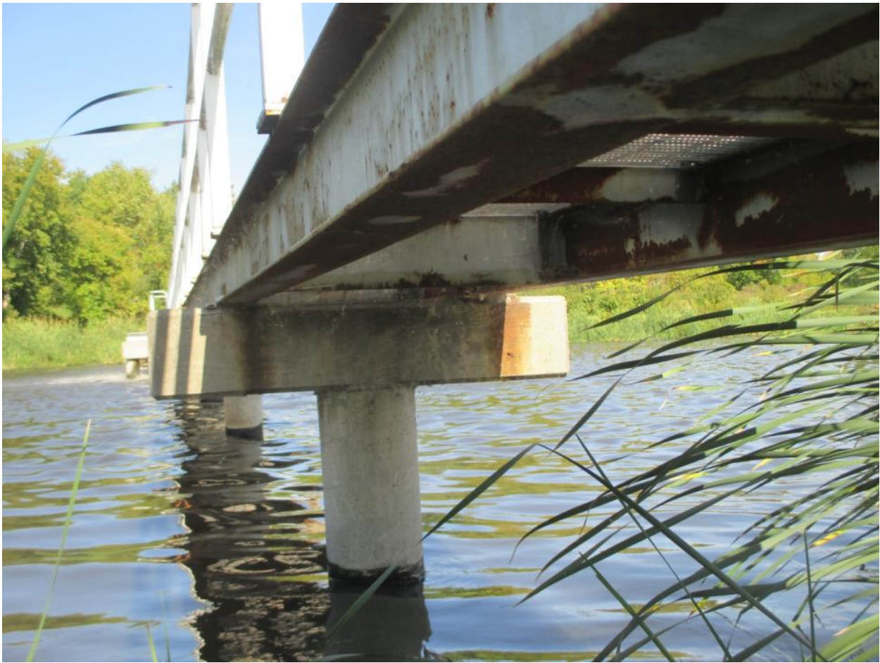
ID02_AS14: Corrosion on Aluminum Walkway
