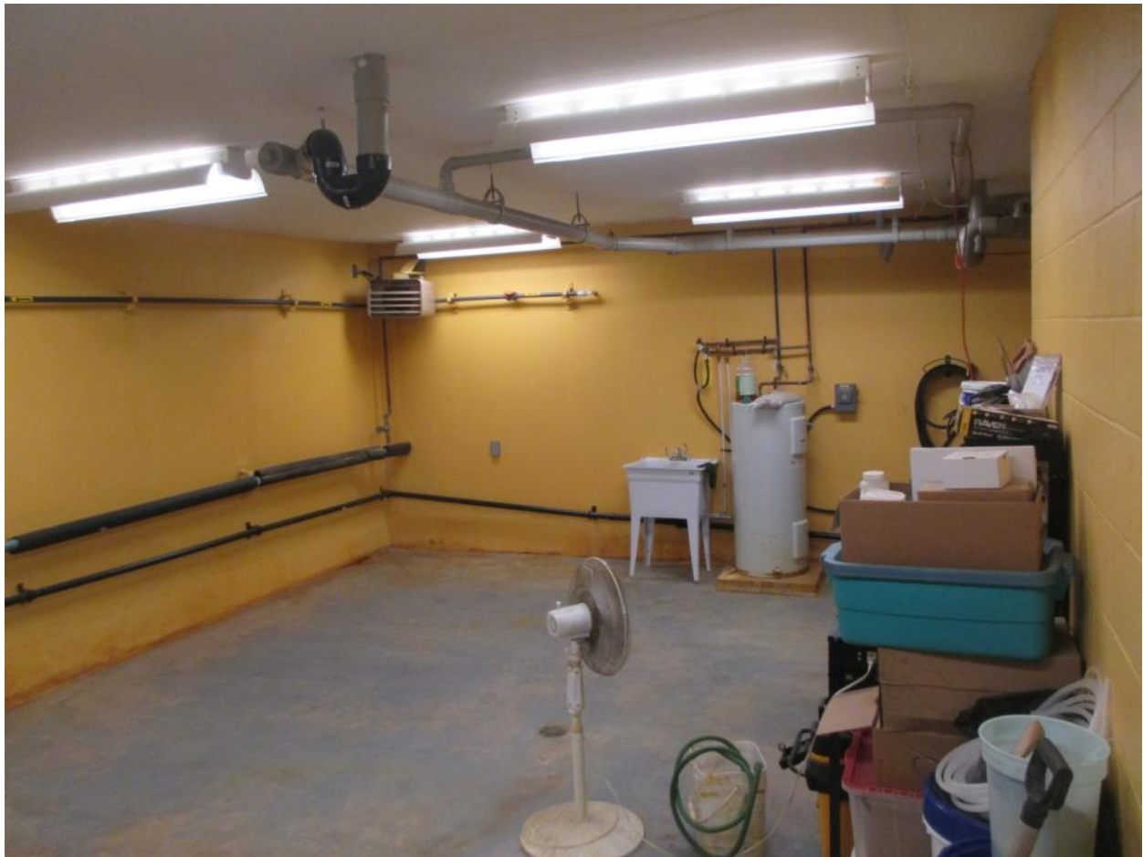
ID02_AS02: Stains on Floor and Walls from Past Ferric Chloride Leak
