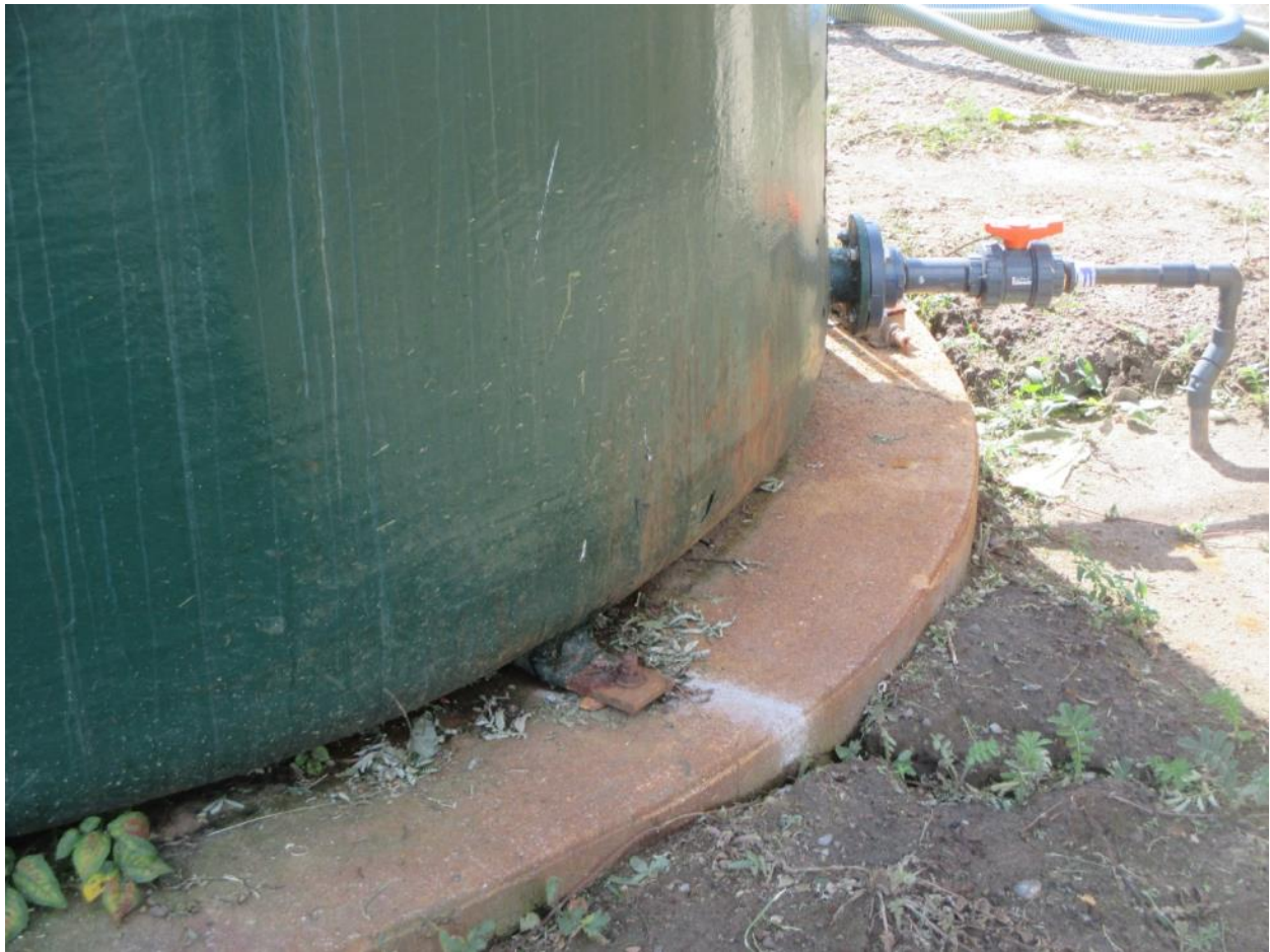
ID02_AS09: Stains from Ferric Chloride Ions
