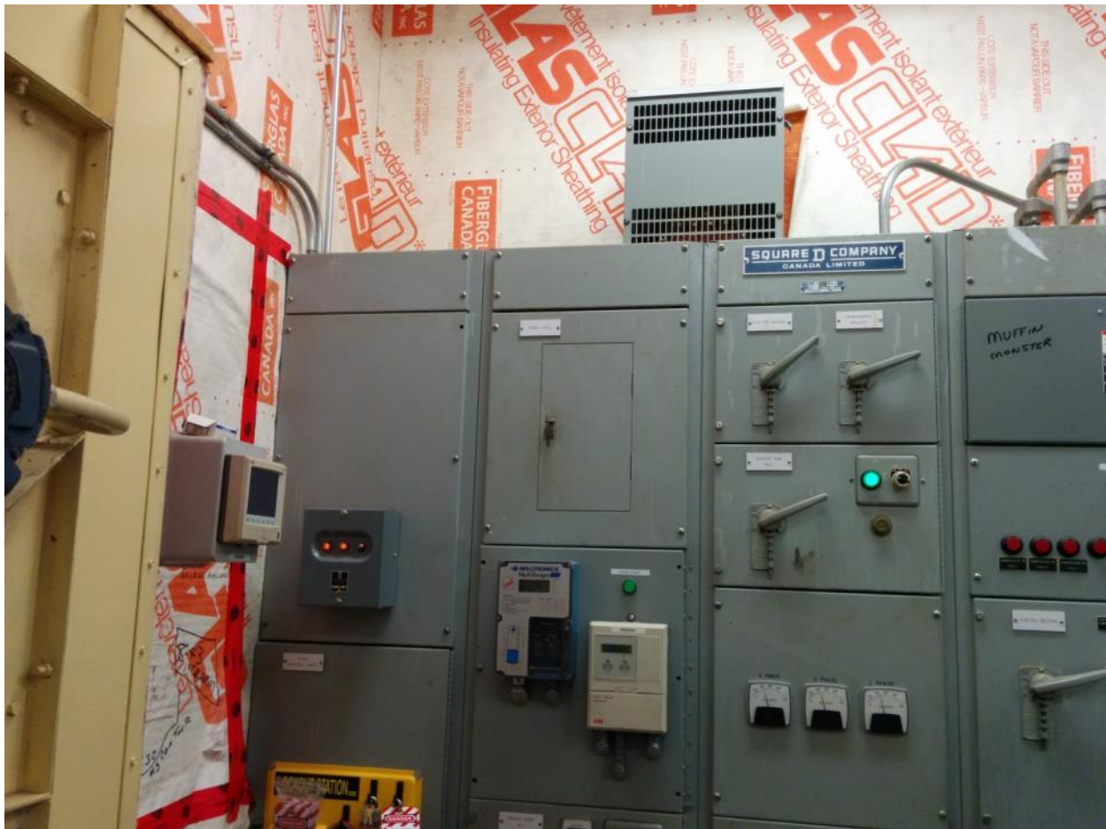
ID01_E01: 120 V Transformer and Top of MCC
