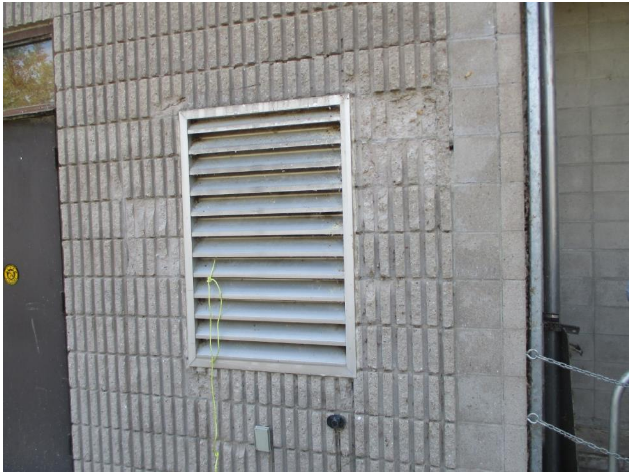
ID01_AS09: Face Shell Cracking and Spalling
