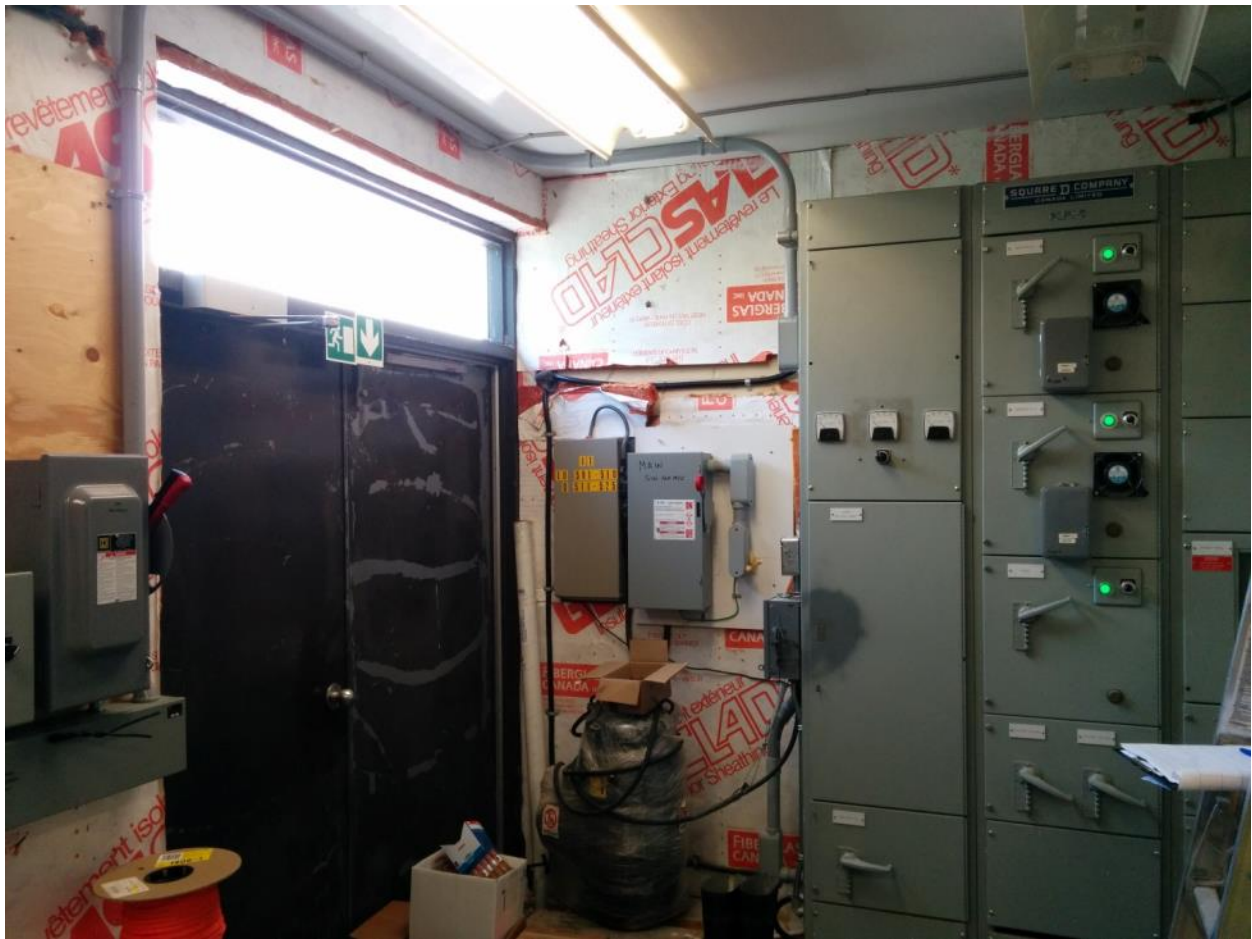
ID02_E03: MCC and Service Disconnect
