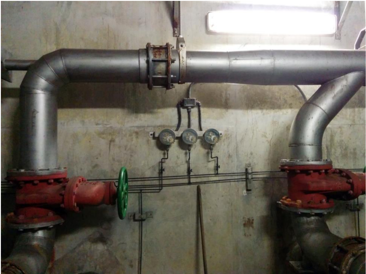
ID01_E05: Pressure Switches
