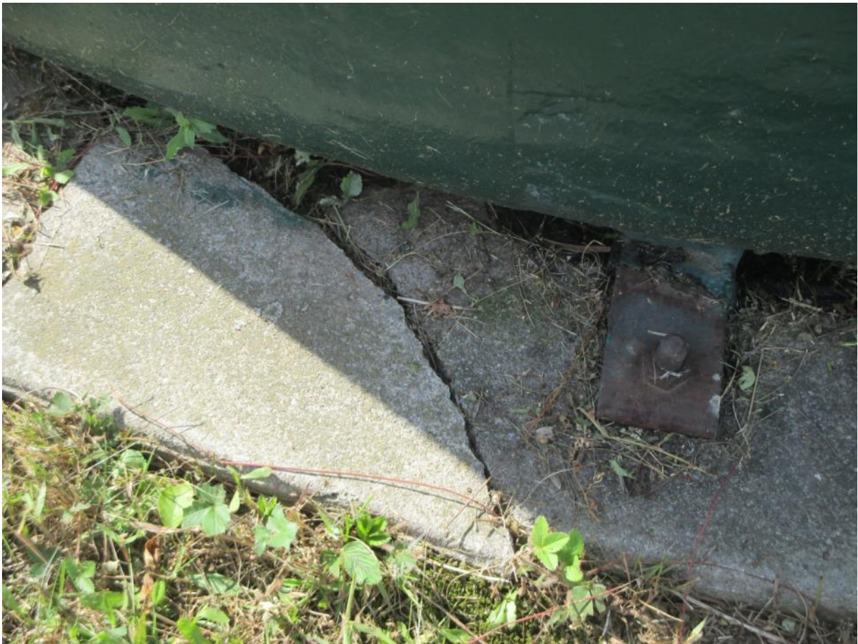
ID02_AS10: Spalled and Broken Concrete Slab
