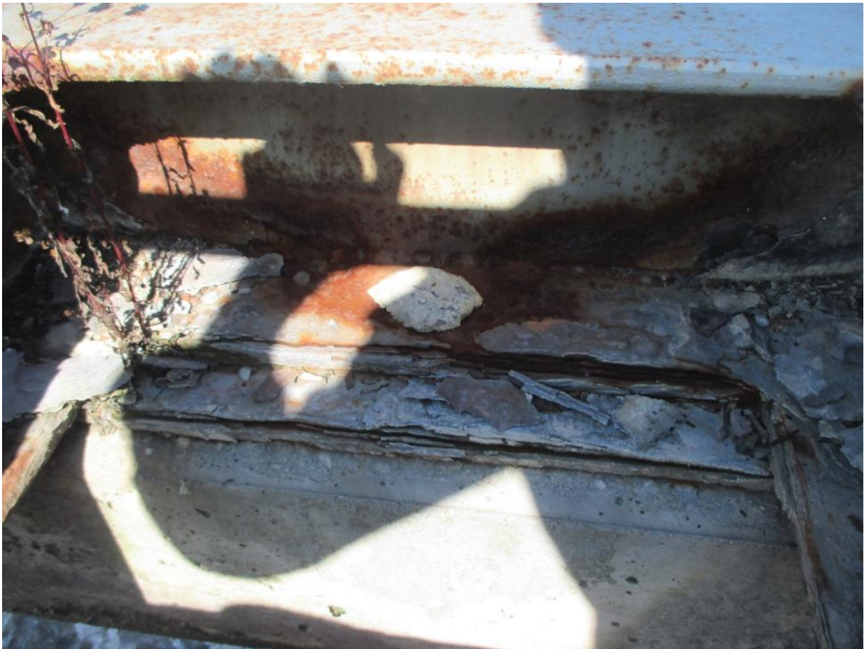
ID02_AS15: Corrosion on Aluminum Walkway
