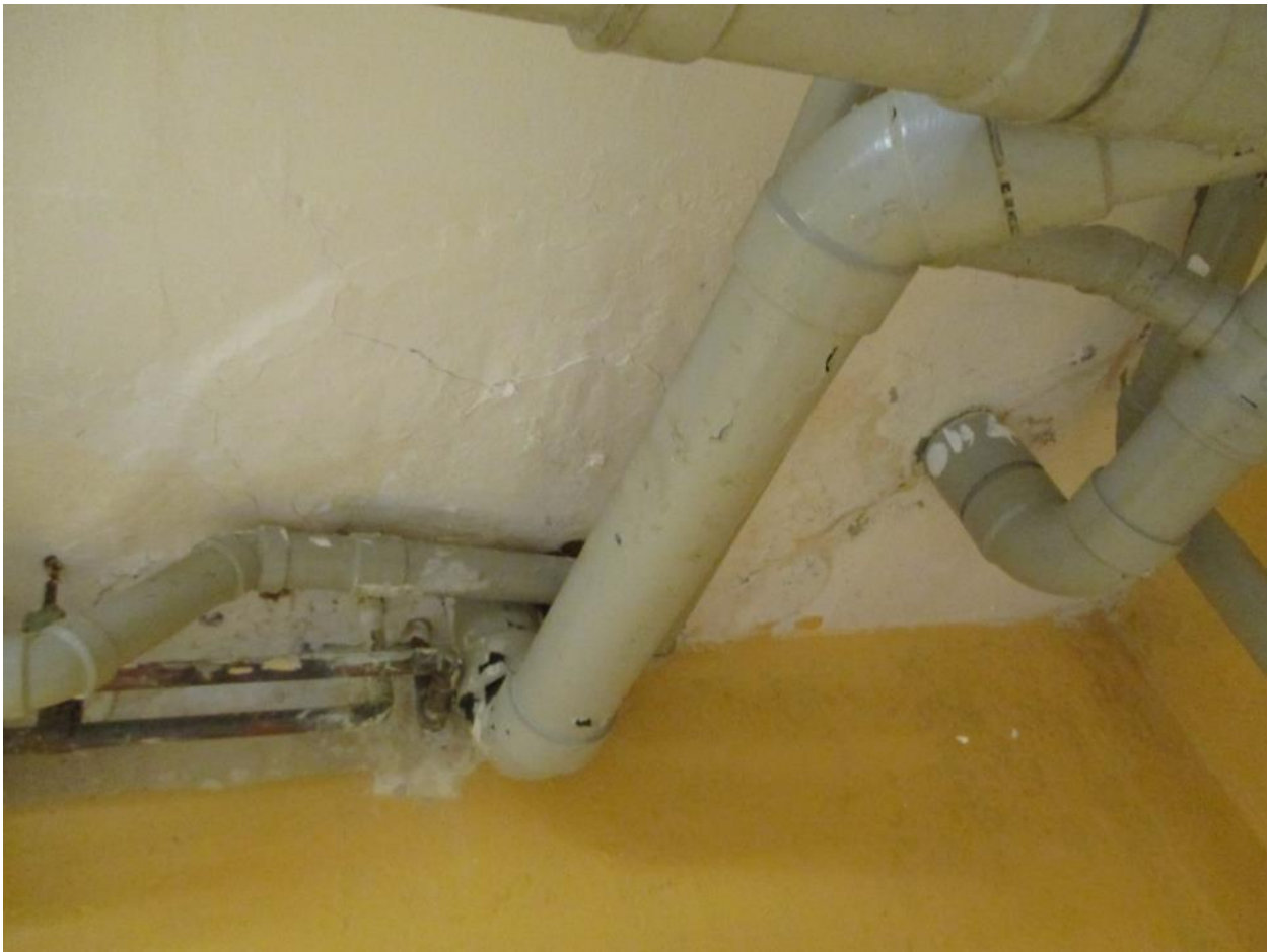
ID02_AS04: Paint Coating Damaged by Moisture
