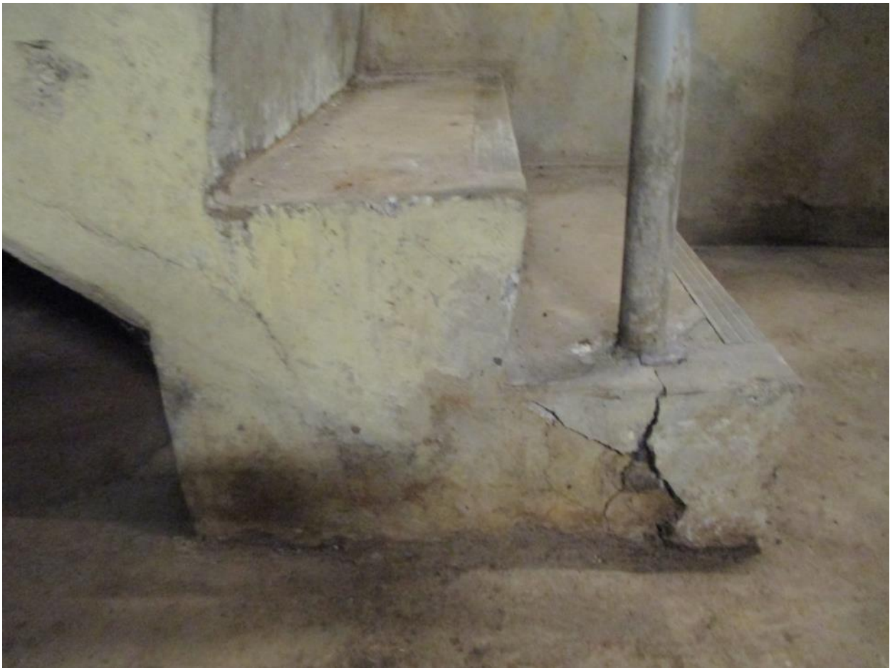
ID01_AS11: Cracked, Delaminated and Spalled Concrete Stair Riser
