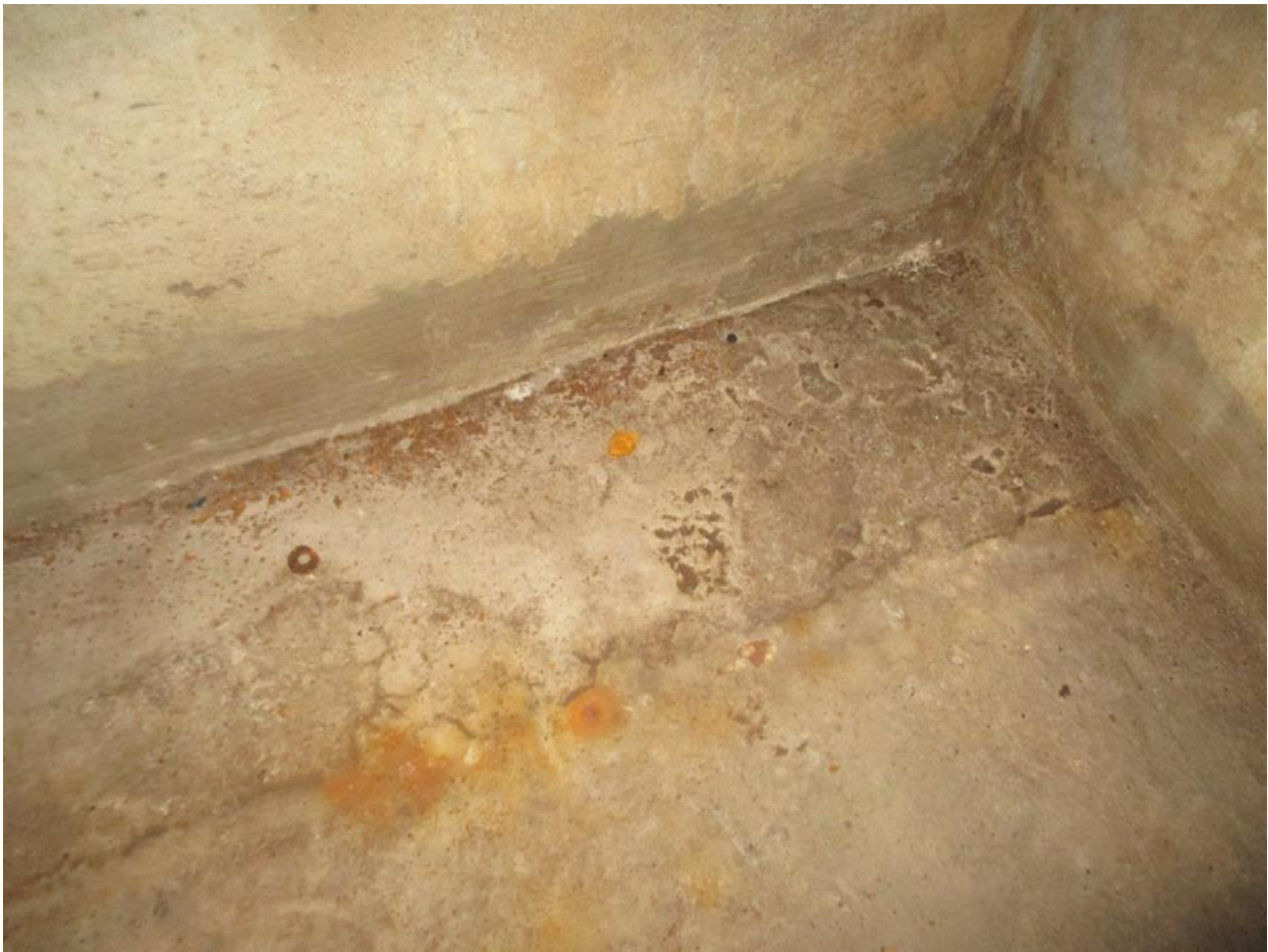
ID01_AS04: Ferrous Staining on Concrete Slab
