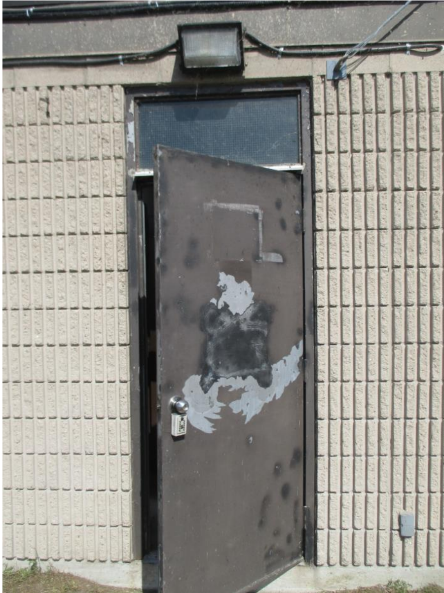
ID02_AS08: Paint Flaking and Chipping from Doors
