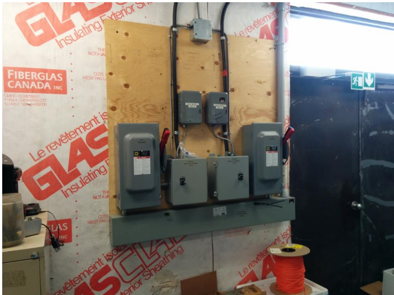
ID02_E02: Starters for New Floating Aerators
