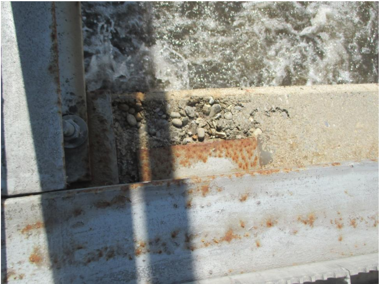
ID02_AS16: Damaged Concrete from Cast-in Plates
