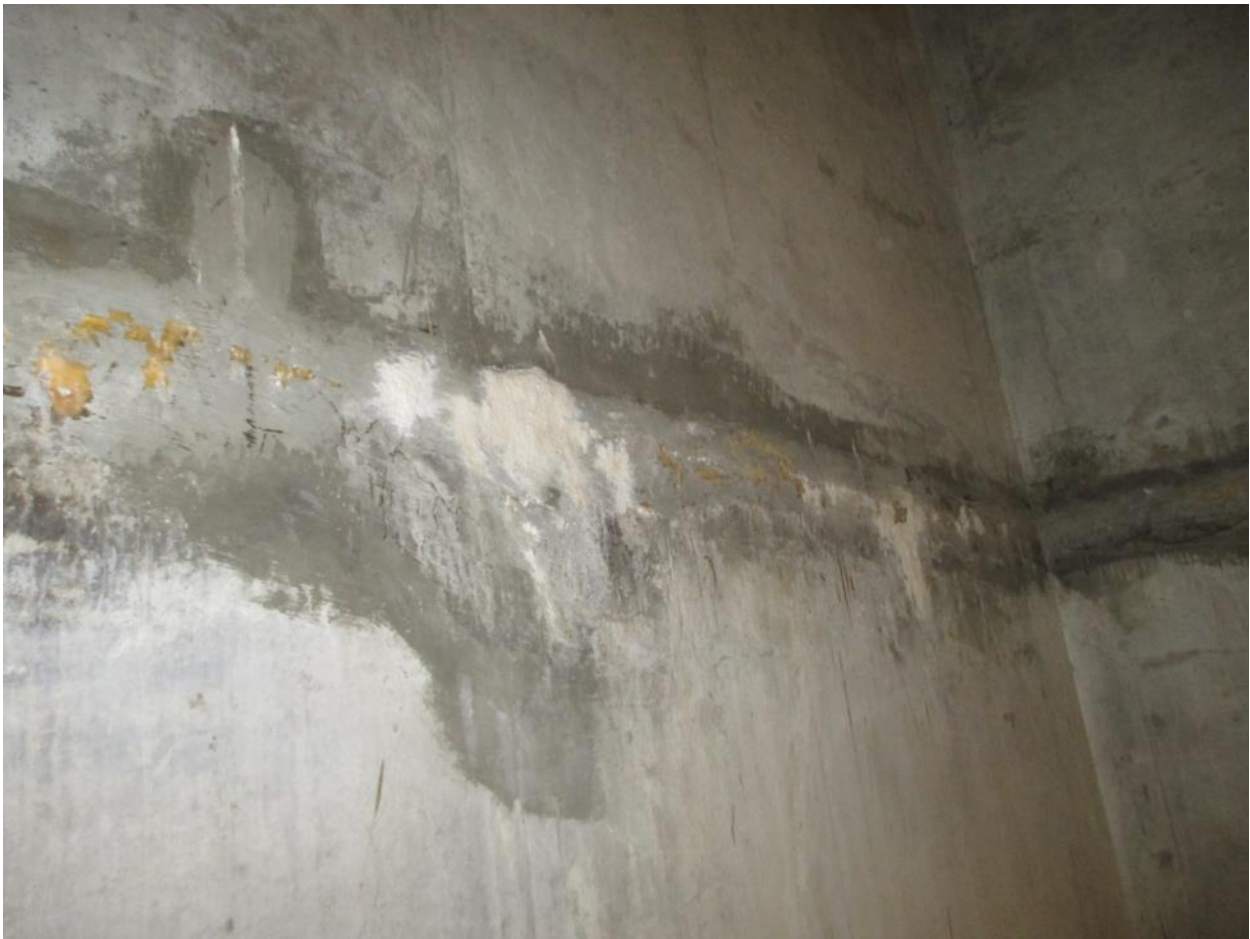
ID01_AS03: Water Damage and Concrete Repairs
