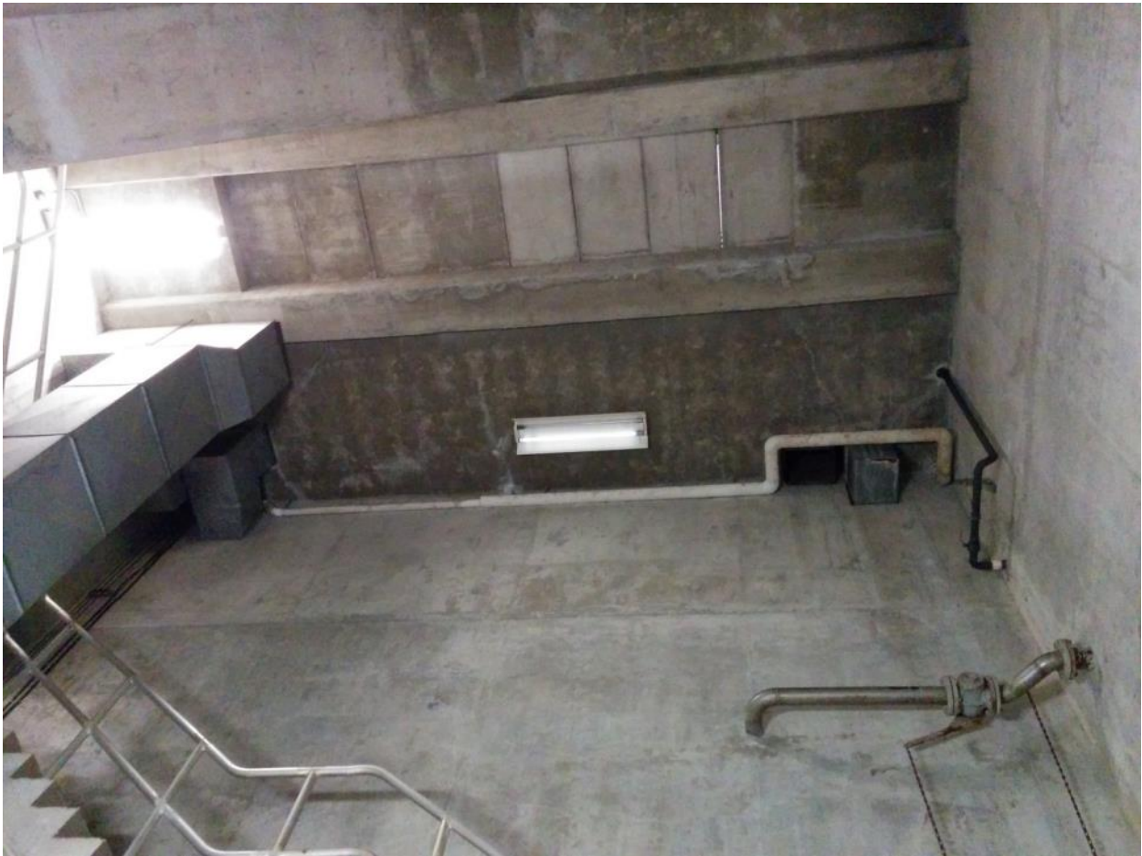
ID01_E02: Inaccessible Light Fixture
