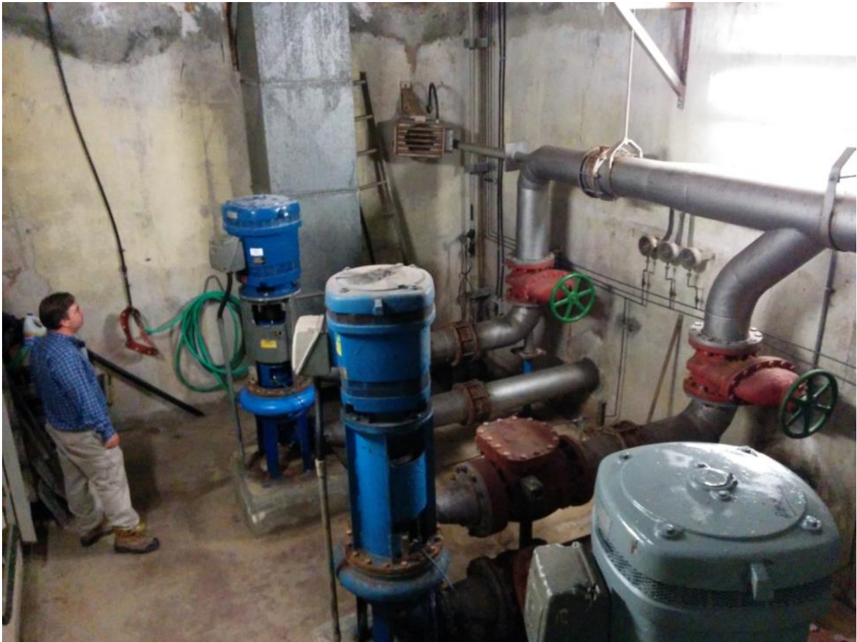
ID01_M03: Raw Sewage Pumps
