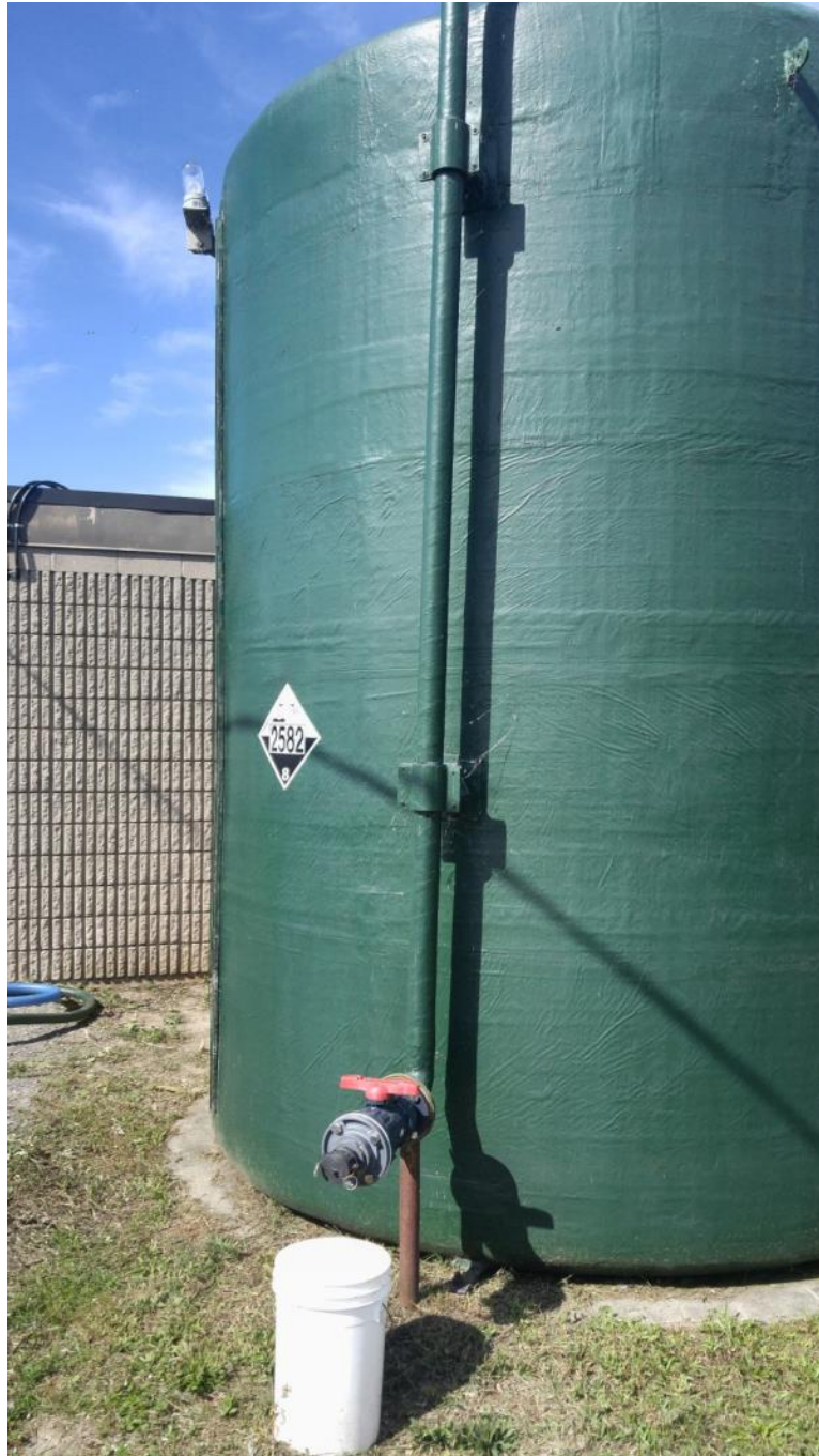
ID02_M03: Outdoor Ferric Chloride Tank
