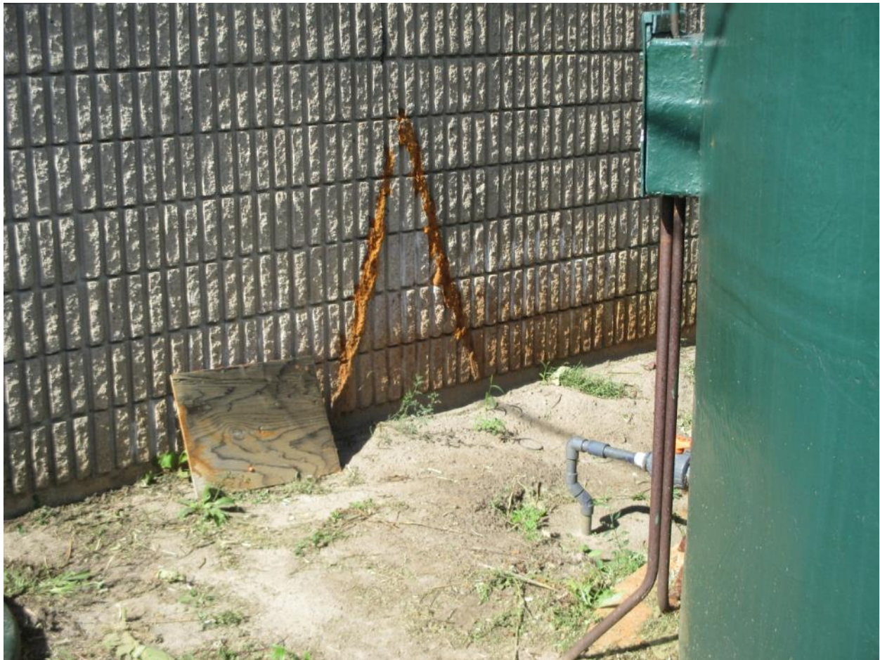
ID02_AS11: Ferrous Staining on Brick
